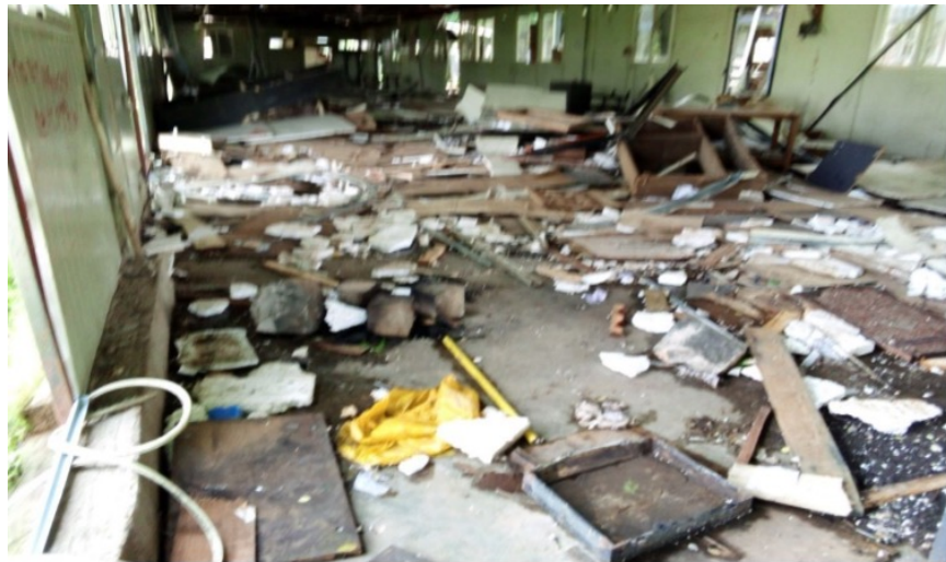
(b) Photograph of Aderkay Polytechnic College after it was looted and shelled by the TPLF forces (Internal View)
